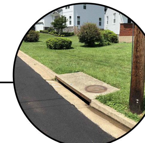
Photo at #1 Elaine Circle. Shrubs will need to be removed. Sidewalk to be built at back of existing utility pole with 4' minimum clearance provided.
