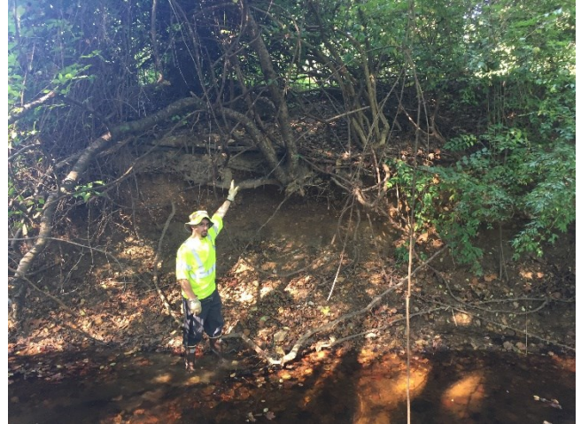
Figure 2. BEHI #8 showing 13' of eroded bank
