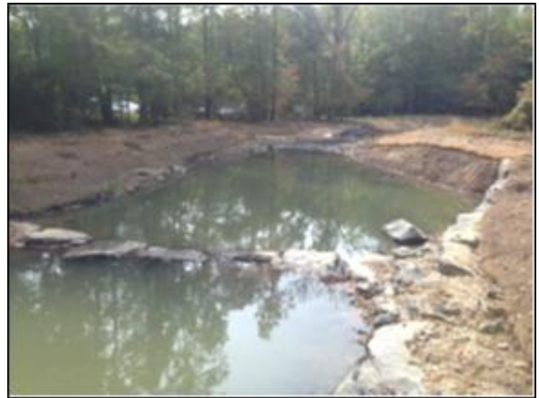
Wolftrap stream restoration during construction. This project is one of the shared credit projects with Fairfax County.
