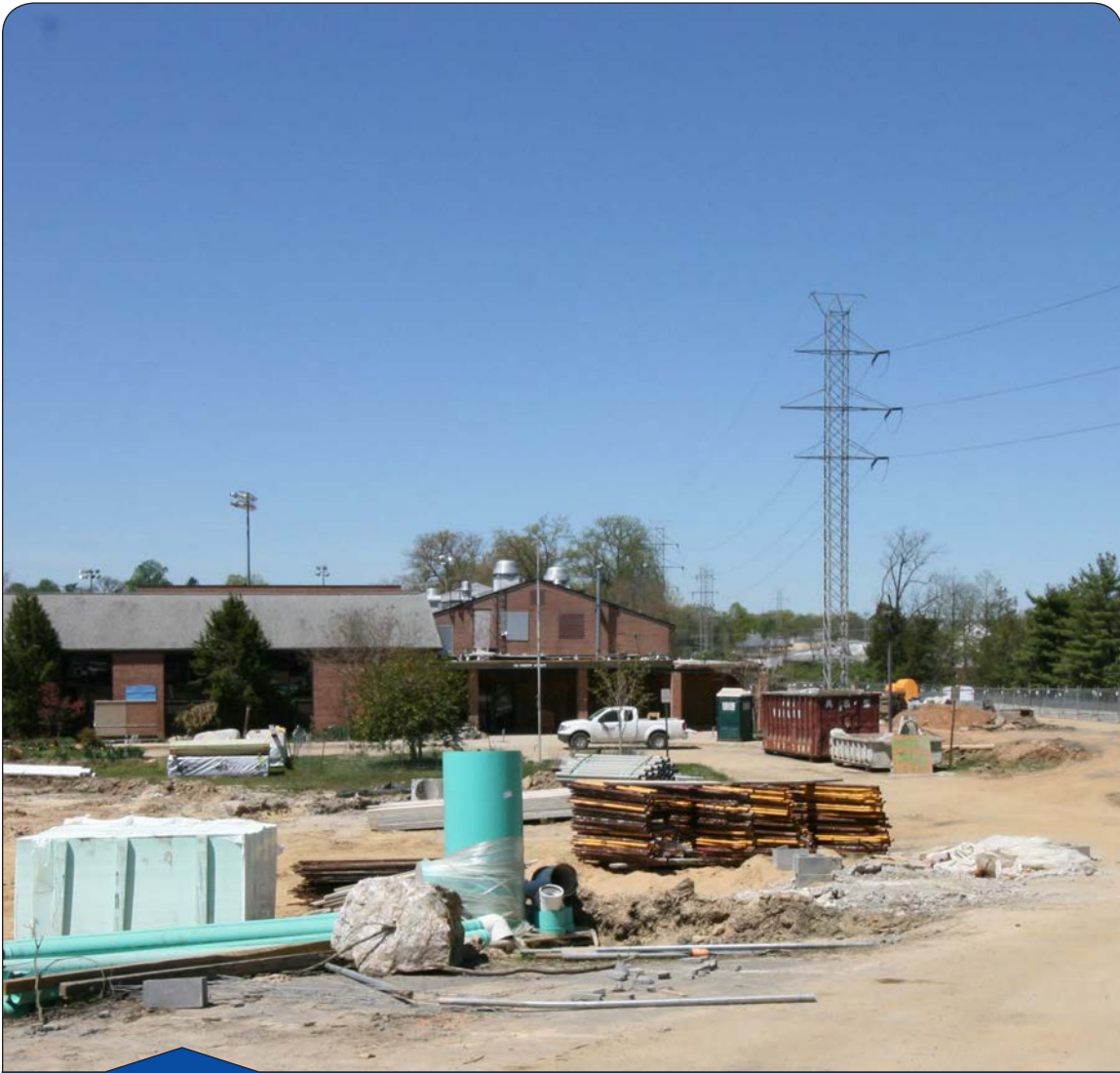
The Community Center is currently undergoing a complete renovation, along with the addition of a new gymnasium towards the rear of the building.
